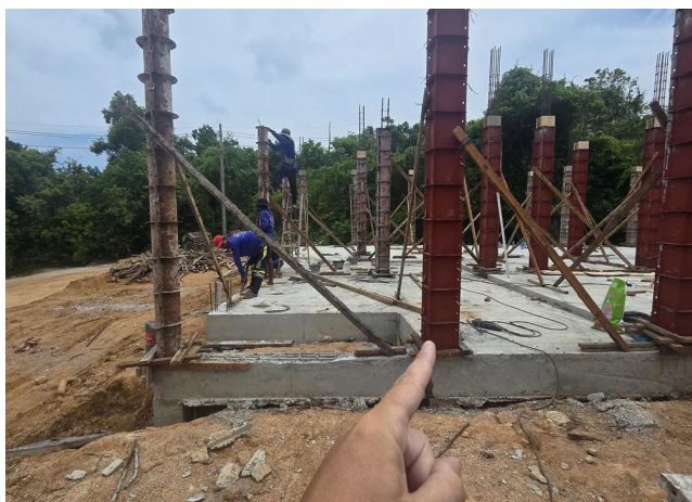
PHOTO 3 Axis C columns after the spacers were corrected
